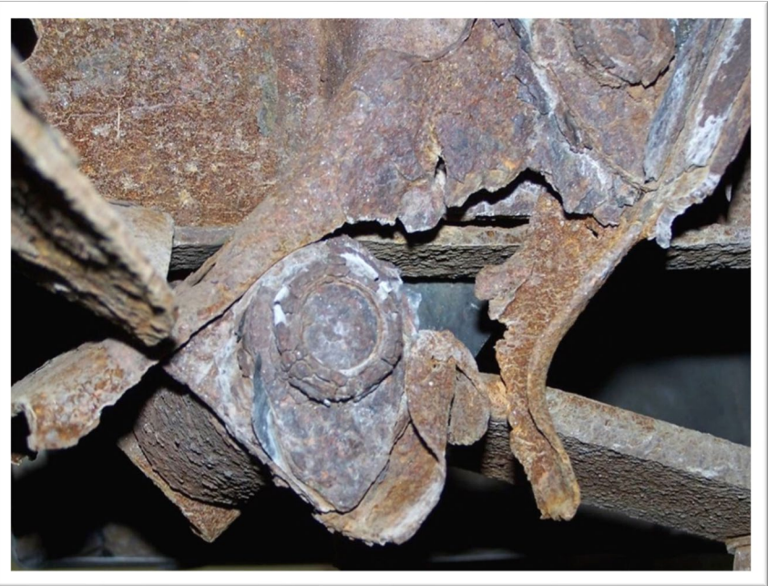
Rotted or broken suspension components
